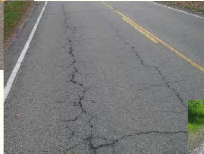
Cracking in Wheel Path
