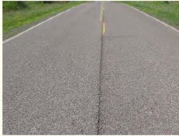
Longitudinal joint cracking
